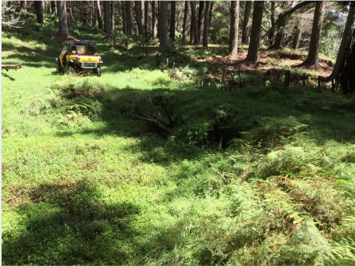
Pic 1: Damaged culvert – Mehrten's Track
