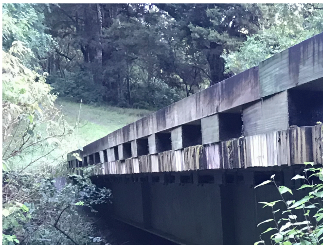
Bridge due for maintenance
