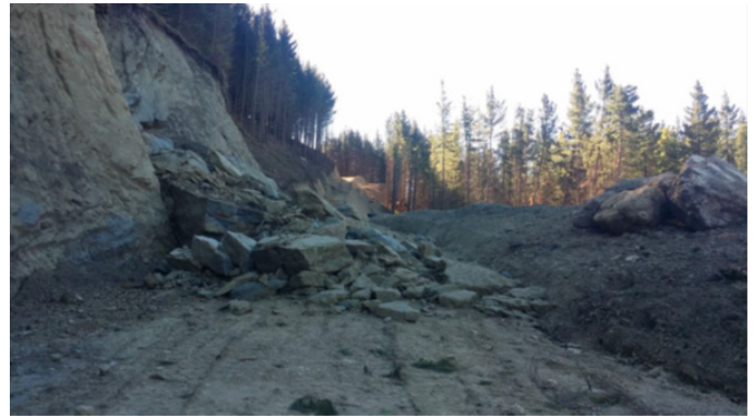
Slip on new road
