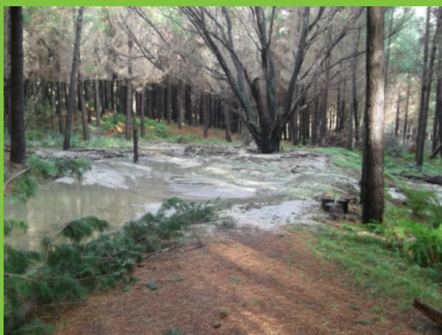
Blocked culvert in Stand 8
