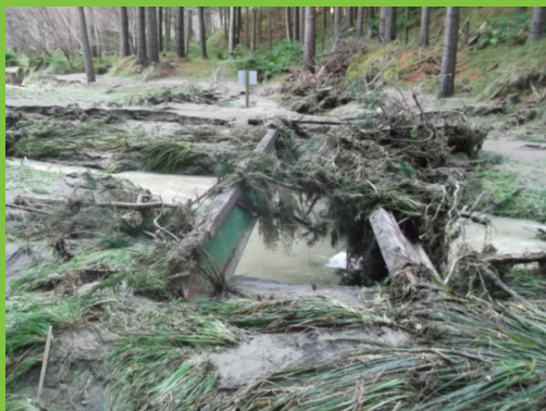
Debris covering what is left of the bridge
