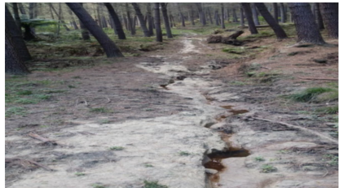
Typical track damage
