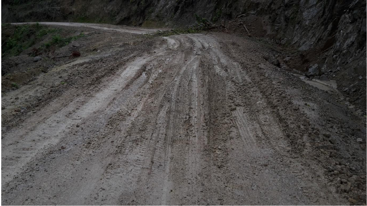
Figure 4: Tyre trail (before), pavement failure, Gillingham Road.
