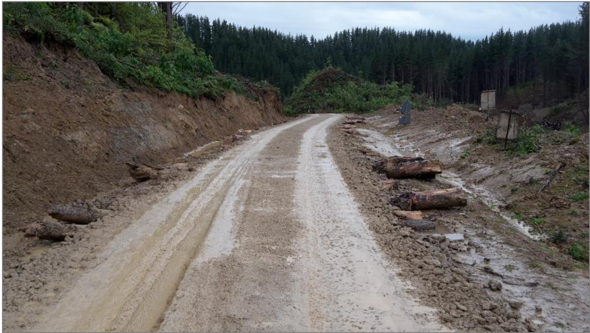
Figure 1: Corduroy used in Farag Rd where pavement failed
