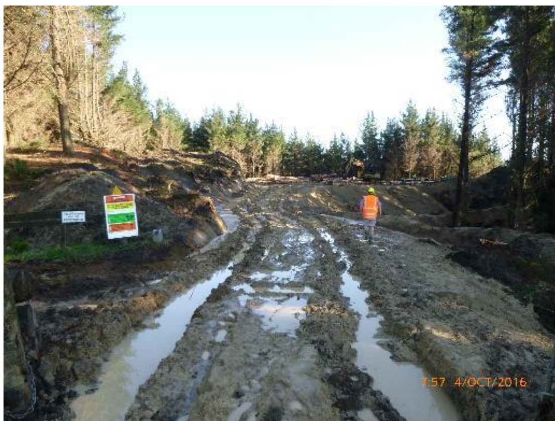
Figure 3: An extremely waterlogged entranceway, preventing any road construction. Note date on Photos.
