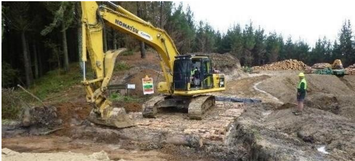
Figure 4: Corduroy entranceway due to very poor soil strength and standing water.
