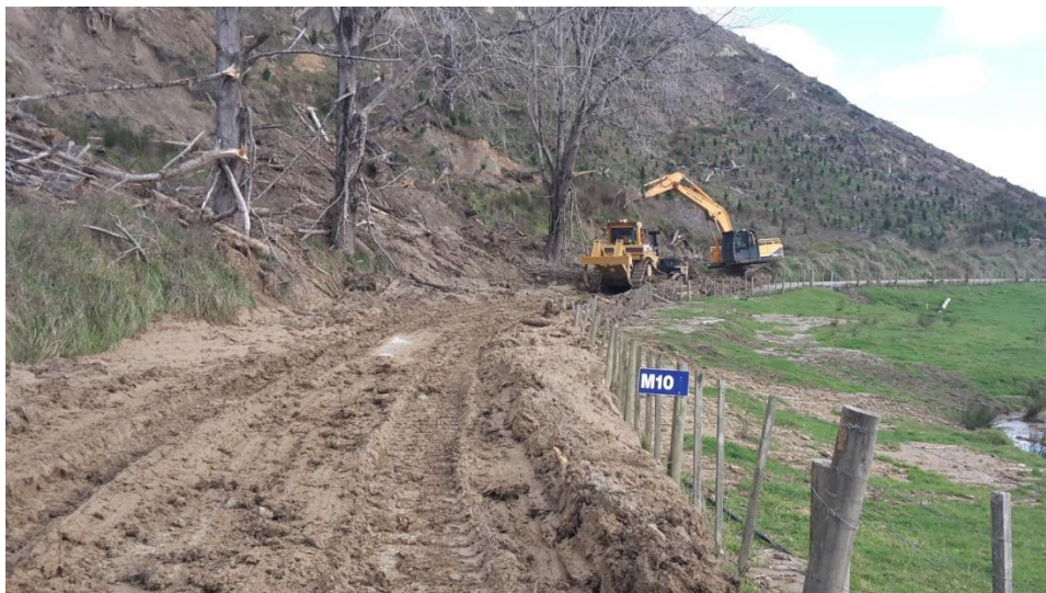
Figure 4 Council section of Waikare Road with slips on to the road.
