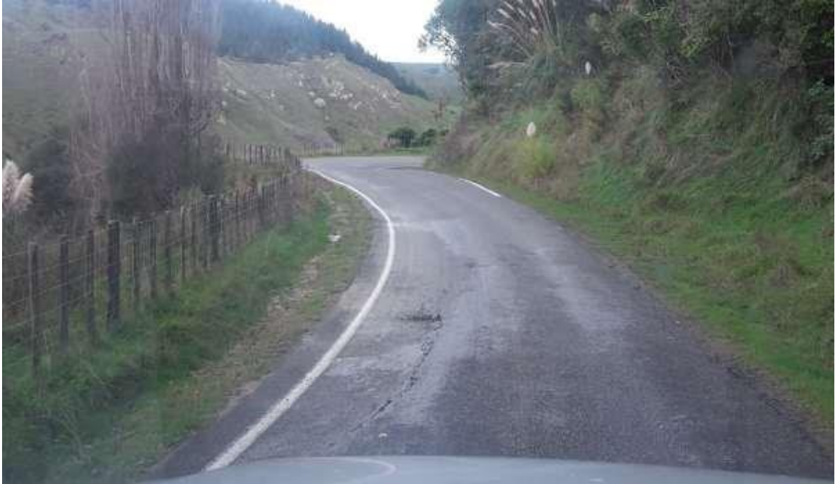
Figure 4 below shows the section of Mangawhio Road showing the development of a crack. Figure 4 (May)
